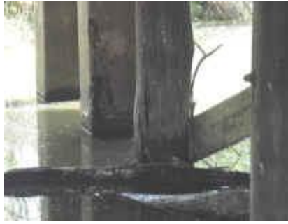
Damaged Timber Pile
