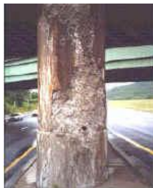
External damage to concrete column
