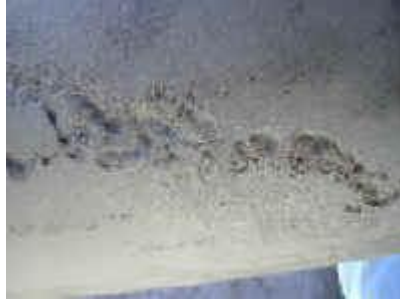
Corrosion pitting was nearly 80% deep
