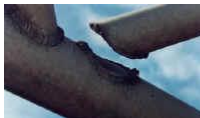
Cracked Weld in Sign Structure
