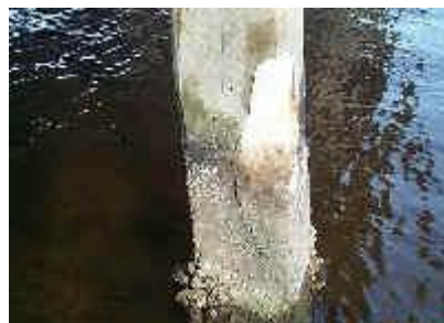
External cosmetic damage to concrete pile
